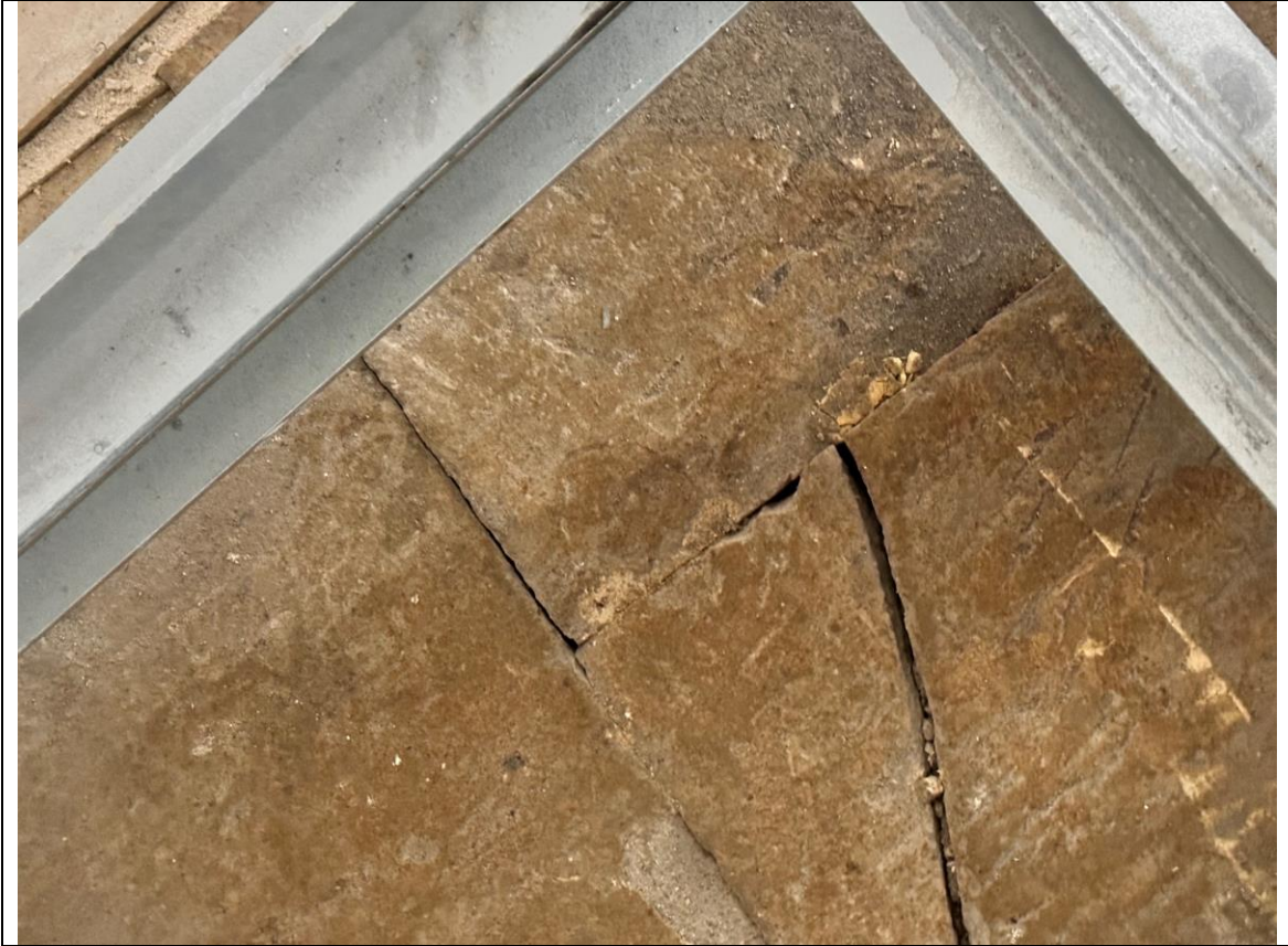
Photo 02-Localised Area with subsided floor
