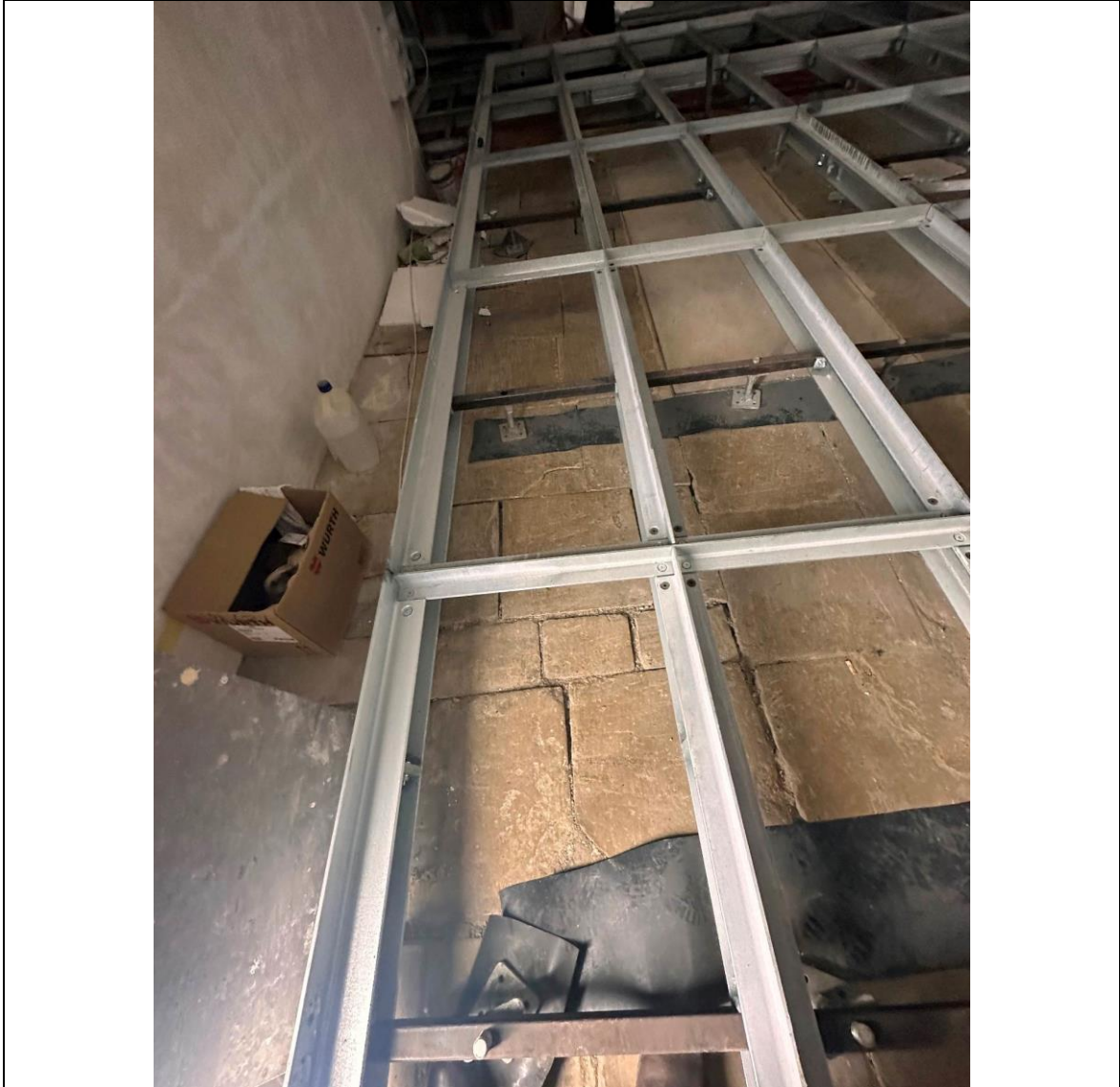
Photo 03-Localised Area with subsided floor
